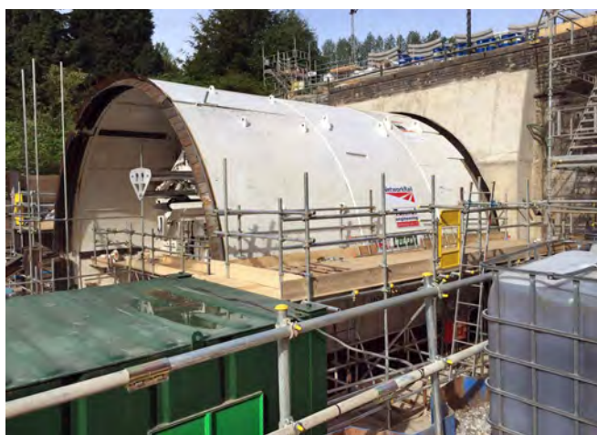
Tunnel Boring Machine 'Fillie' in place on 24 July 2015. Photo from Network Rail
